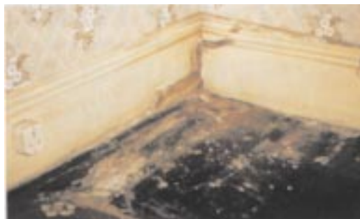
Dry rot attack in building
