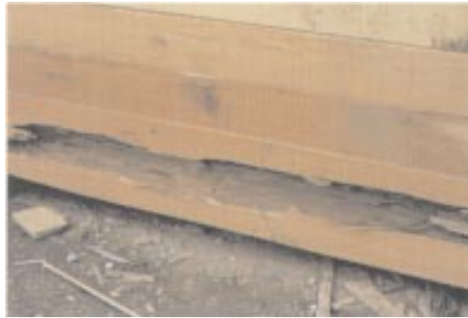
Termite attack in building timbers
