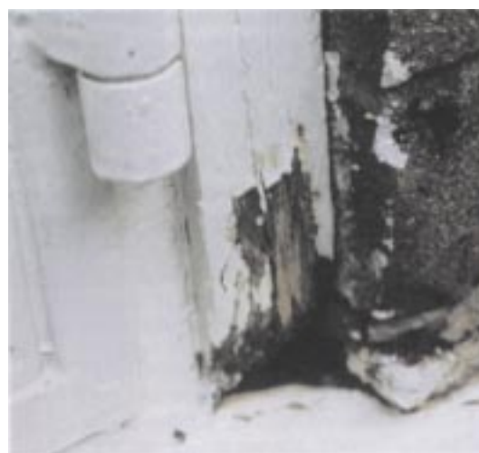
Wet rot decay in window joinery due to poor detailing between the sill and brickwork
