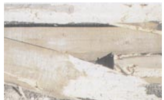
Damage to softwood roofing timbers by the house longhorn beetle
