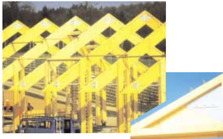
Figure 7 I beams and columns fabricated from Kerto-S LVL for a tied portal frame structure. Warehouse in Freising, Germany. Photo: STEP
